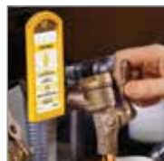
Frame houses labels on Bulk Systems
